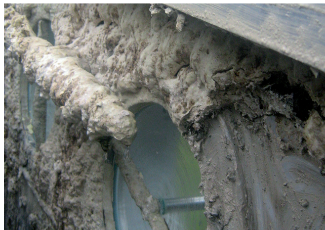
Figure 3 Build-up of sulfur inside a biodigester, as a result of desulfurization
